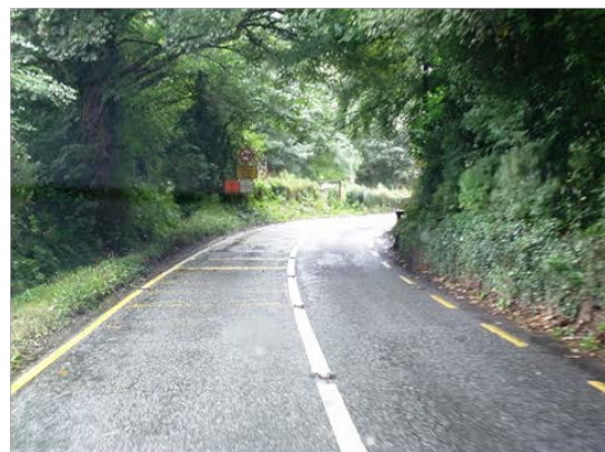
Existing L1015 with tight bends and poor visibility
